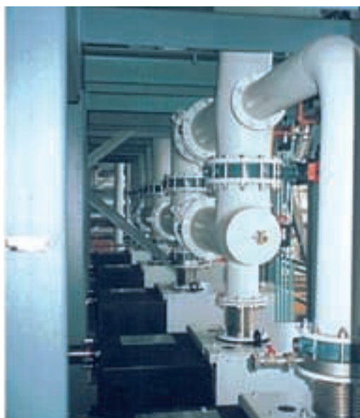
Vacuum pump system of a continuous freeze-drying plant
