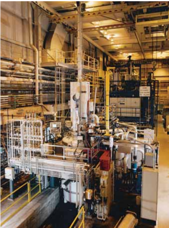
VIM-IC 10 DS/SC/LMC for the Pilot Production of large DS/SC Components using LMC Process
