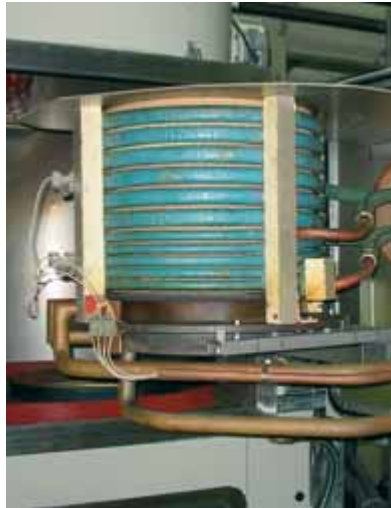
Induction Mold Heater attached to Furnace Door
